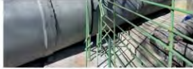
Photo 2: Cutoff wall reinforcement. Note cutoff wall will be at mid-span of RCP.
